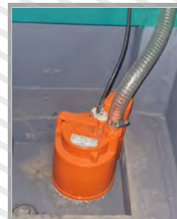
Water Transfer Pump Exuded water is transferred back into the system for suspended solids removal
