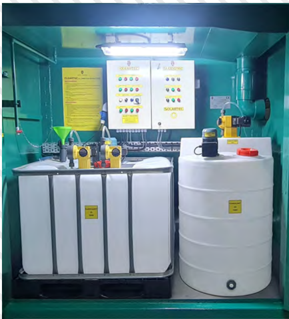
Chemical Dosing Chamber
