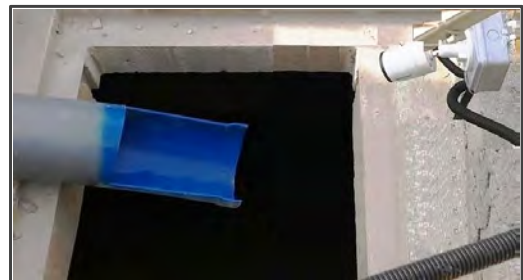
Typical CCTV Installation adjacent to public drain
