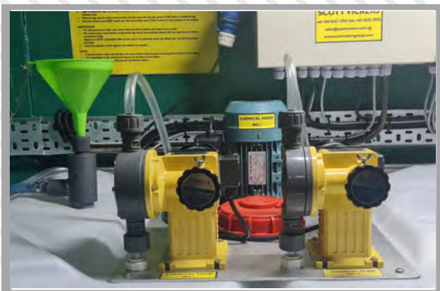
FI Dosing Pumps & Mixer
