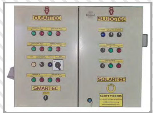
Control Panel for automatic operation of:-
