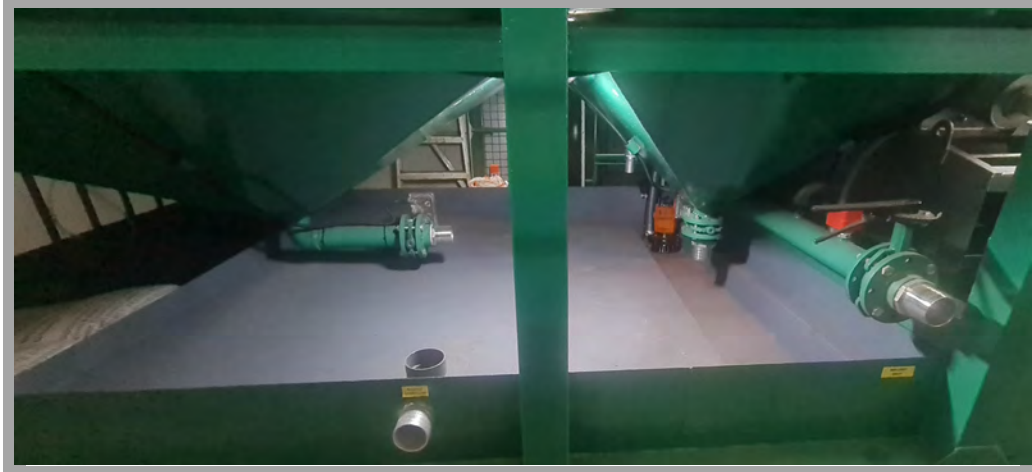
Liquid Sludge Collection Chamber with Auto Desludge Valves & Overflow
