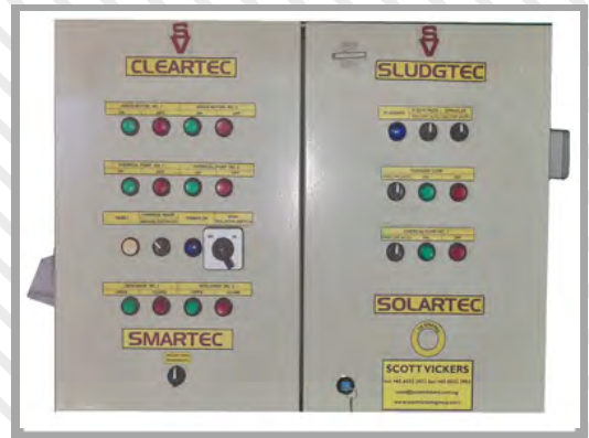
Control Panel for automatic operation of:-
