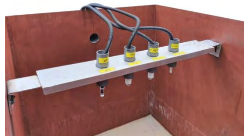
Monitoring Probes in Collection Tank
