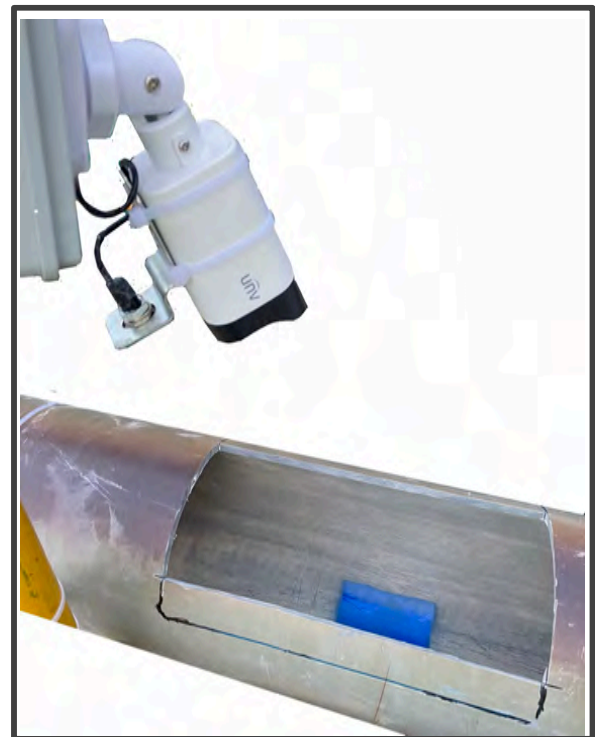
CCTV System complete with LED light and blue marker in Discharge Pipe
