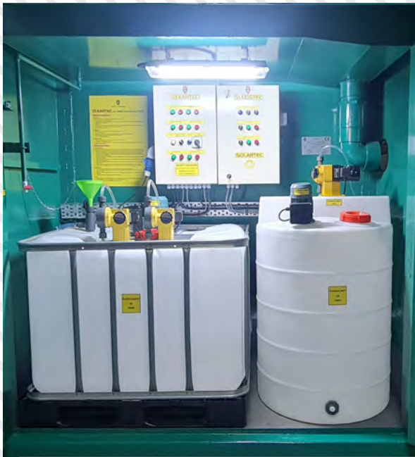
Chemical Dosing Chamber
