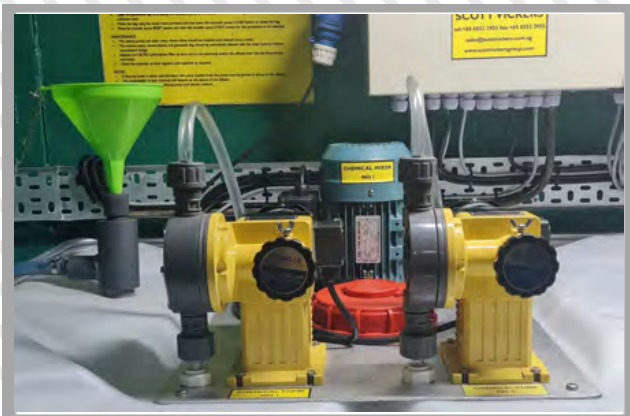
FI Dosing Pumps & Mixer
