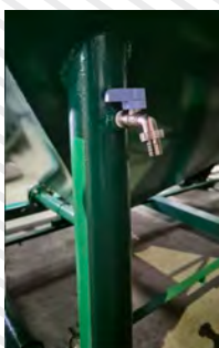
Primary Chamber Sampling Point to verify chemical mixing quality
