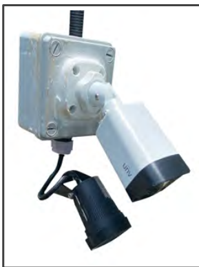
CCTV System complete with LED light
