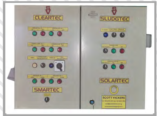
Control Panel for automatic operation of:-
