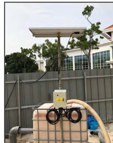
Typical TSS Monitoring Installation with Solar Panel on top
