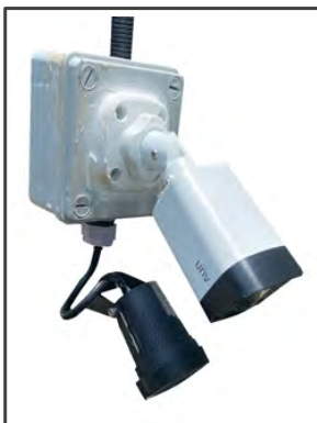
CCTV System complete with LED light
