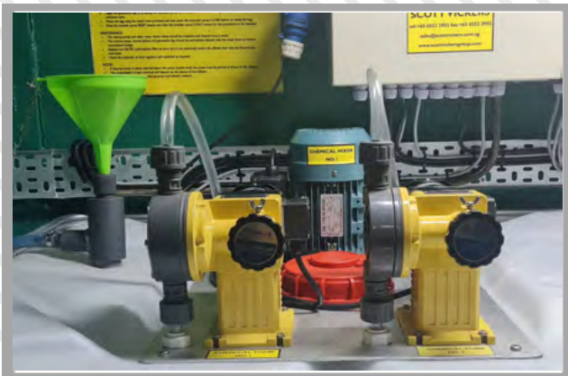
FI Dosing Pumps & Mixer
