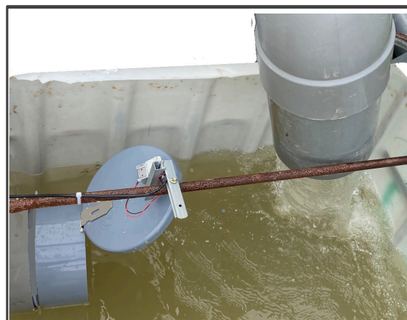
Automatic Discharge Control
