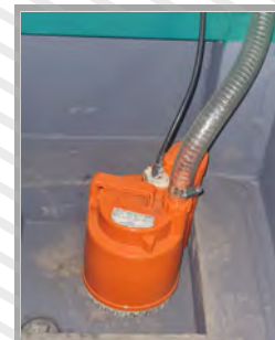
Water Transfer Pump Exuded water is transferred back into the system for suspended solids removal
